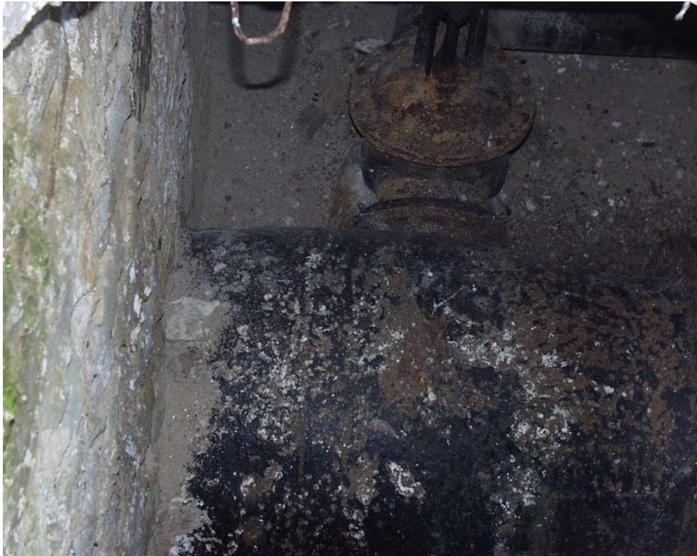
Picture 2 Water pipe
