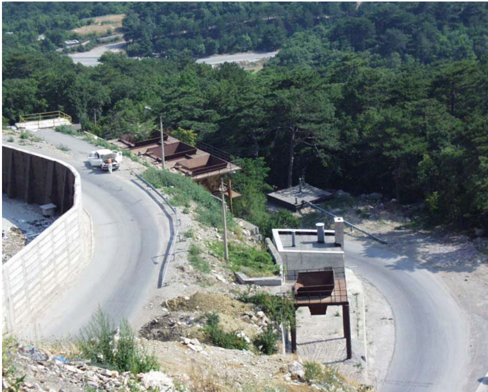
Picture 52 Yalta Landfill: Hoppers for waste transfer
